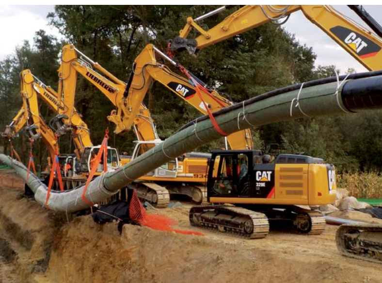
Pipeline Cover France, 2014, durable protection and buoyancy prevention for Artère de l'Adour gas pipeline using Incomat Pipeline Cover system.
