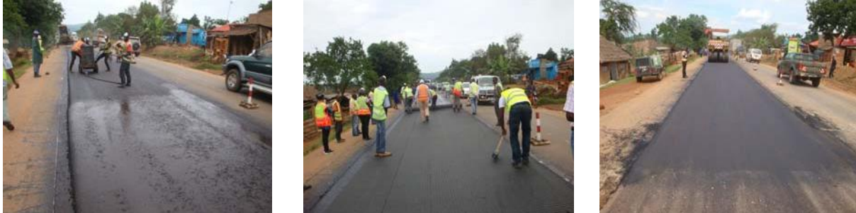
Figures 14a, 14b and 14c: Work steps; spraying of bitumen emulsion, installation of polyester asphalt reinforcement grid and overlaying with 5cm asphalt
