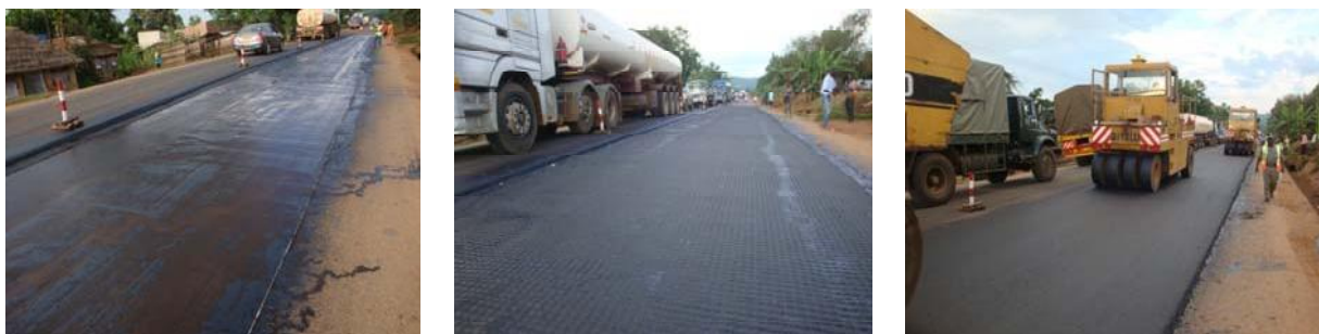
Figures 15a and 15b: Spraying of bitumen emulsion 0.7 kg/m 2 , installation of polyester asphalt reinforcement grid and overlaying with 7cm asphalt
