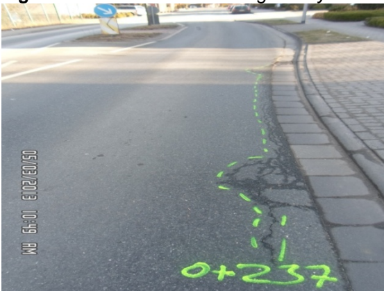
Figure 6. Cracking resulting from road works
