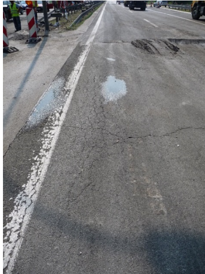
Figure 8. Reflective cracking from cement stabilized base
