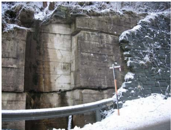
Fig. 2 Damage to retaining walls along "old" route
